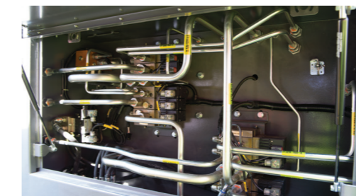
Steel pipework for better heat dissipation
